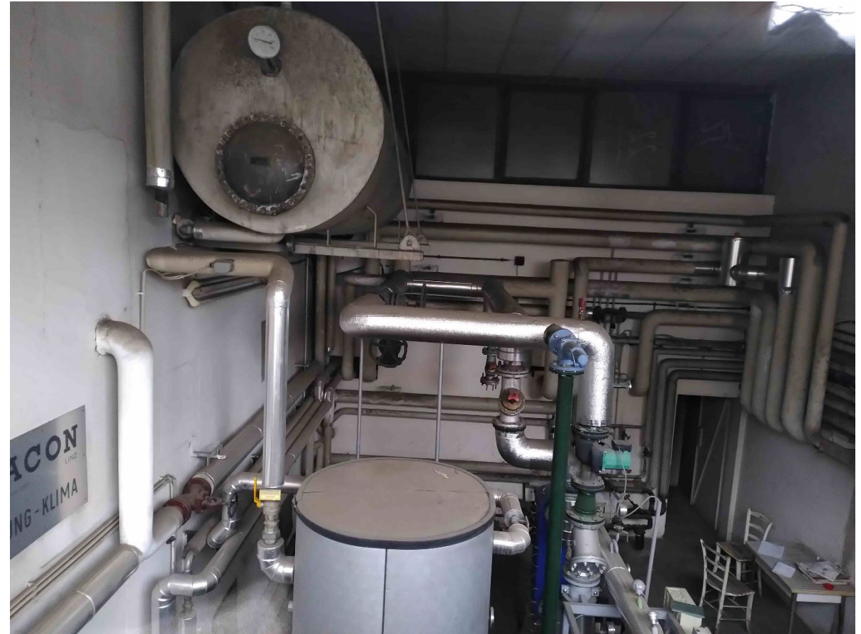
District heating station
